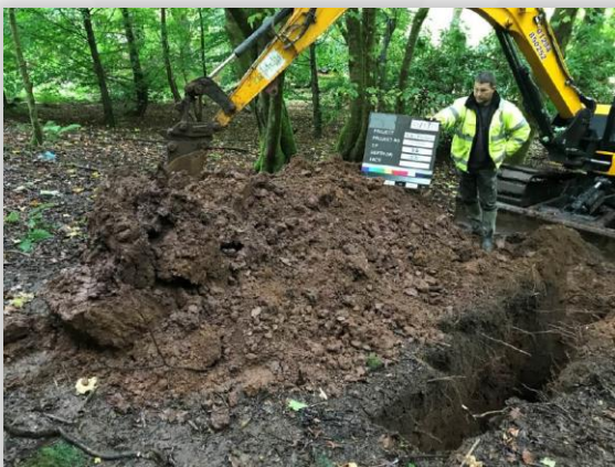
Trial pitting underway at location TP36 in the south-east of the site.
