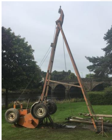
Cable Percussion rig working close to the site of the Battle of Stirling Bridge
