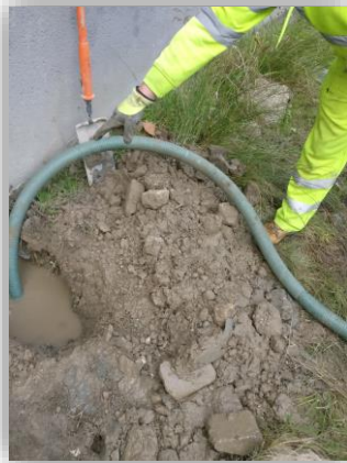
Groundwater encountered during hand pit excavations caused some difficulty progressing the excavations
